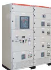
Main Low Voltage Switchboards
